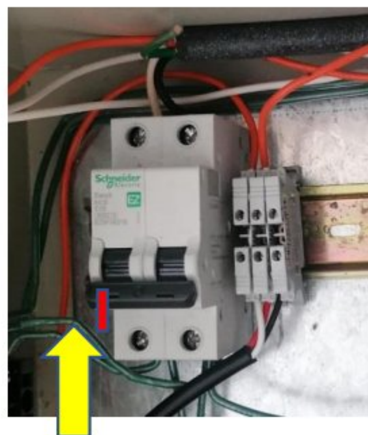
Figura 2: Control del breaker principal
