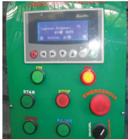
FIGURA 3.60 TABLERO DE CONTROL
