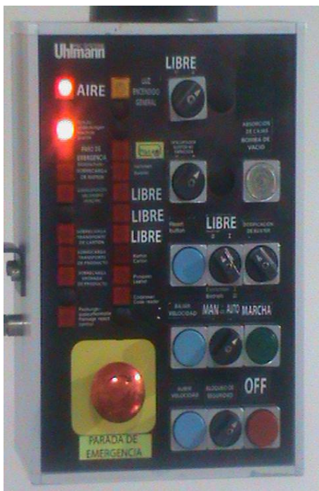
Panel de control.
