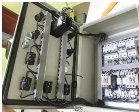
Figura 16: Tablero de control
