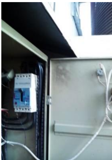
a) Interruptor principal
