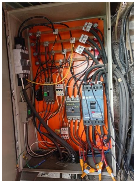
Figura 4.9 Tablero principal (TP-B).
