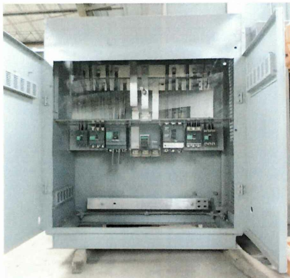
Figura No. 3.16 Tablero 220 V
