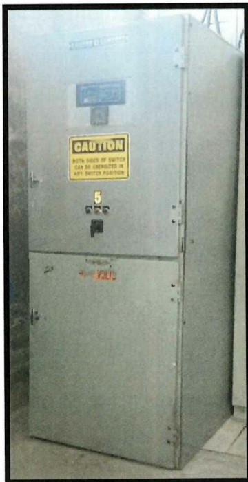
Figura No. 2.2 Interruptor Square-D
