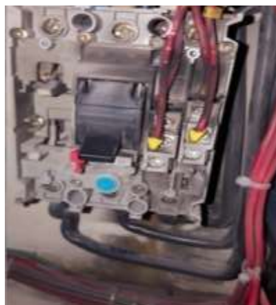
Figura 3.8 Cortocircuito Bracker principal bomba P1121 D
